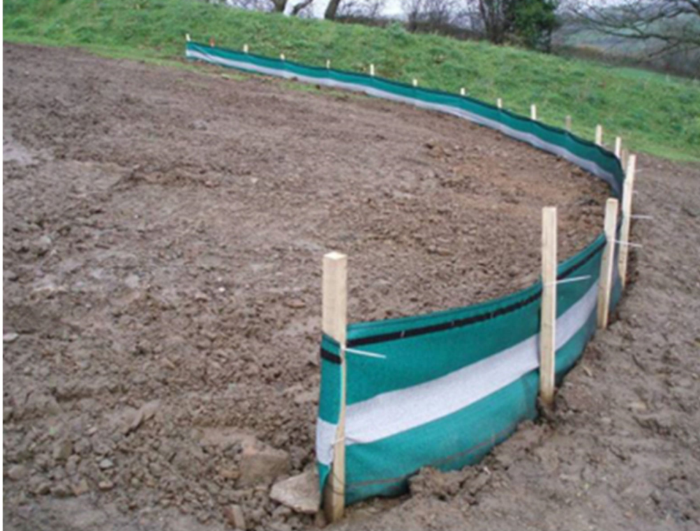
Plate 7: Typical silt fencing
