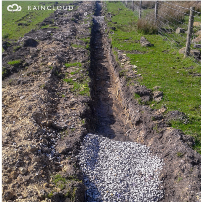
Plate 8: Check dam example
